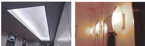
LED lighting being used at the Sanix Hakata Building
