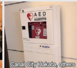
Canal City Hakata, others AED installation
